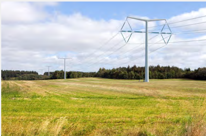
We will use T-pylons for most of the route
