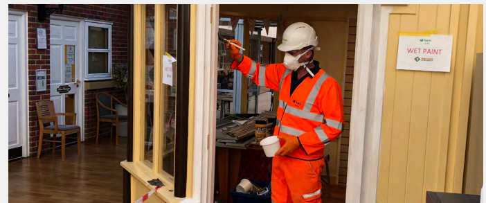
Frazer Hodgkins, hard at work putting the finishing touches to the carpentry
